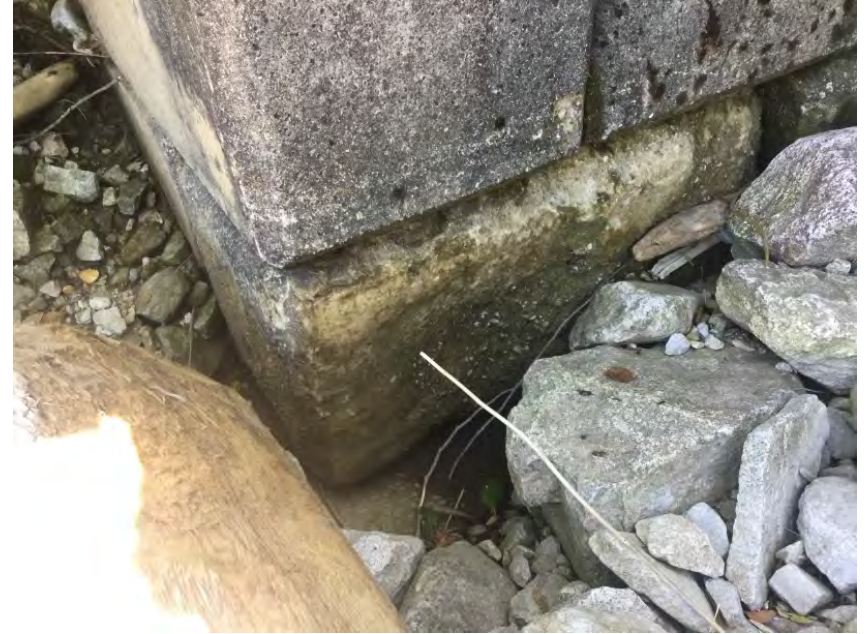
Spalling of Bottom Lock Block at Downstream Left Abutment
