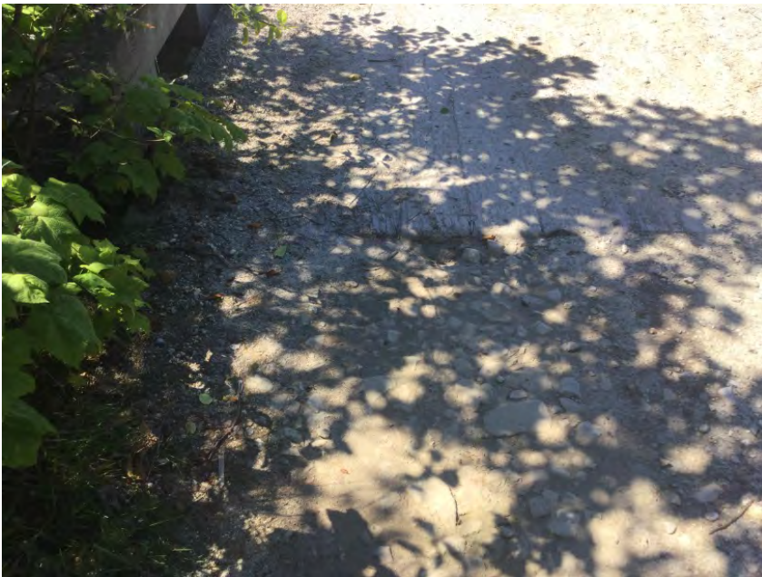
Pothole in Approach with Worn Wearing Planks
