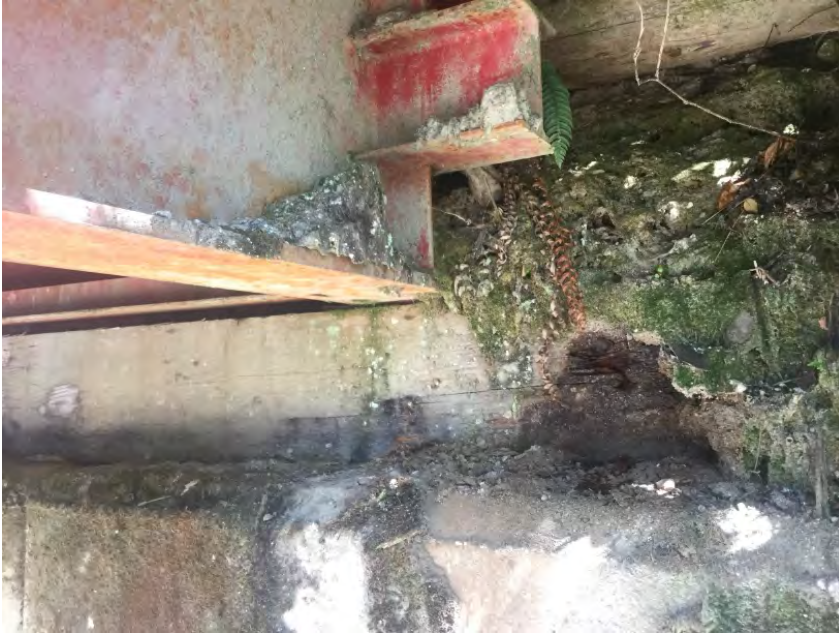
Right Abutment Rotten Sill
