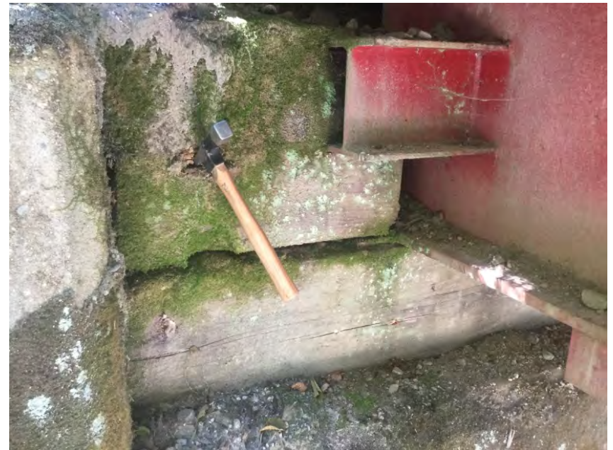
Left Abutment Rotten Ballast Wall
